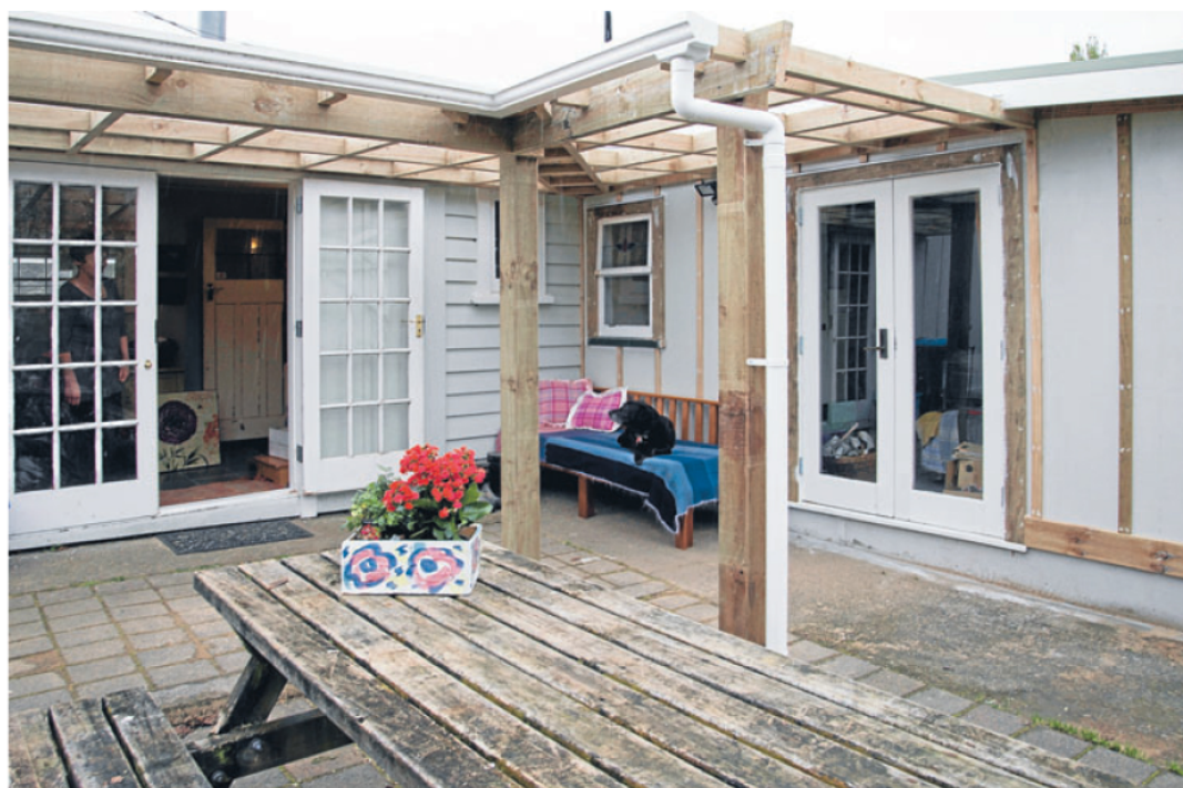
Exterior update: The Edwards reclad the exterior of their home in board and batten, removing a cladding builder Trevor Taylor, of Smith & Sons, suspected had an element of asbestos.
